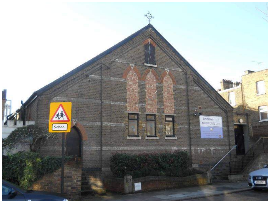
Bricking up of windows on Addison Boys Club has harmed the appearance of this elevation on Redan Street.
