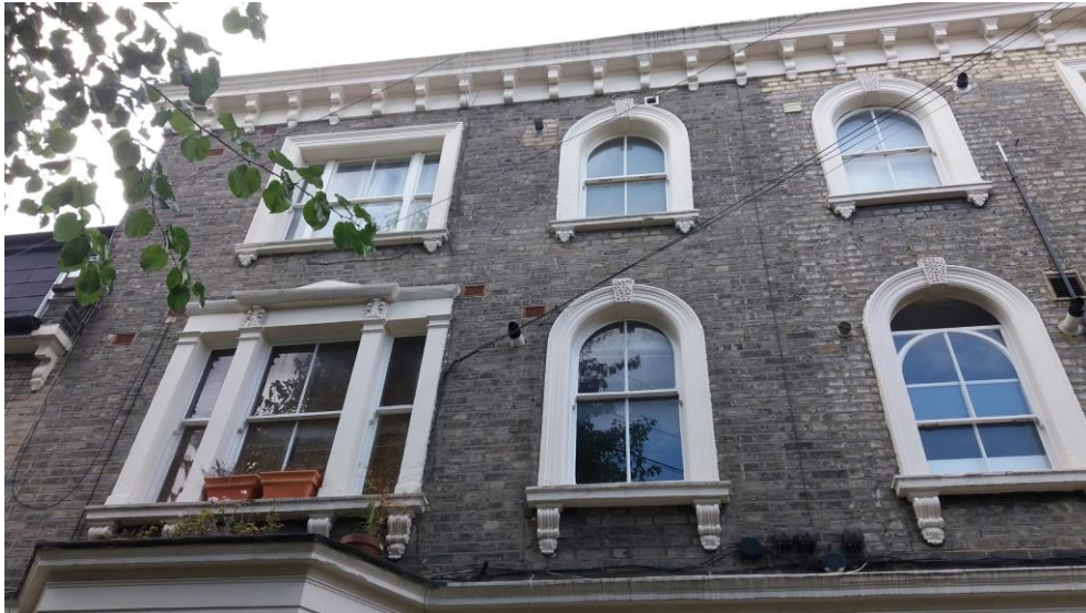
Deep cornices with moulded modillions. An original feature of nos. 2-10 Barclay Road. Missing on 2 & 4.
