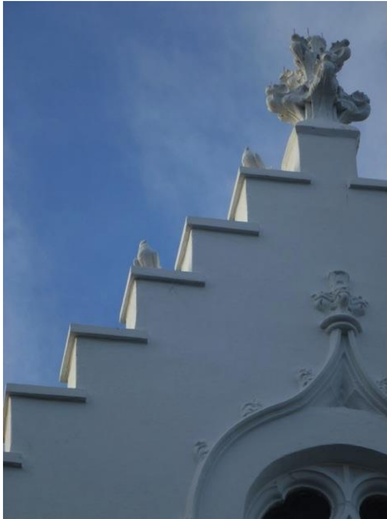
Former St. John's Hall – detail of gable showing finial and plaster pigeons.
