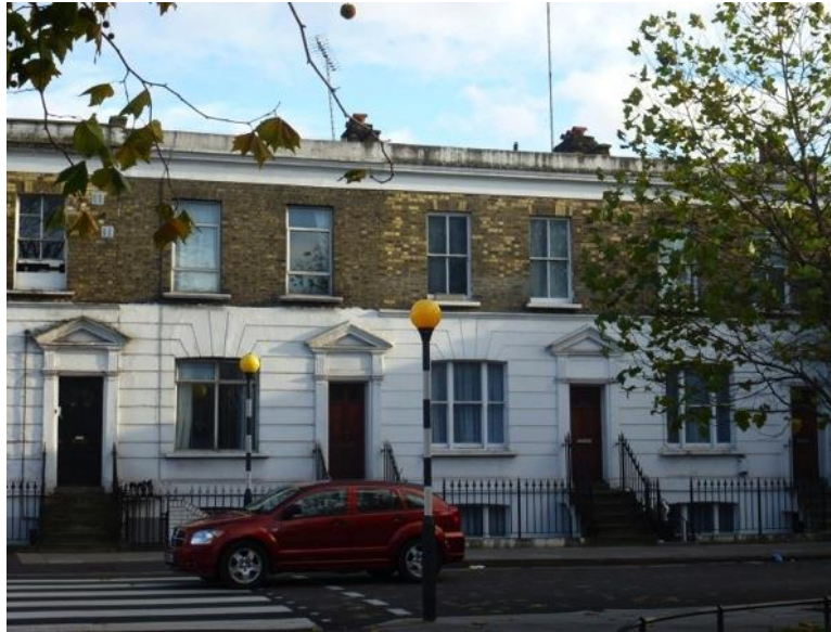
Nos. 34-44 Studland Street; the character of this almost uniform terrace is compromised by unfortunate alterations to windows.
