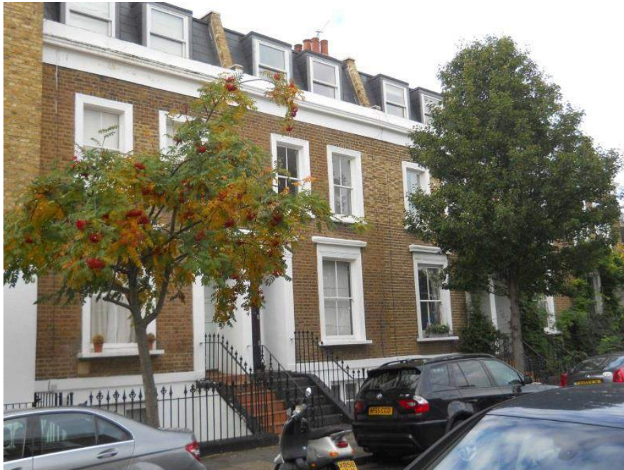
Recessed mansard roofs nos. 5-13 Masbro Road. Street trees and planting in narrow front gardens enhance the street scene.
